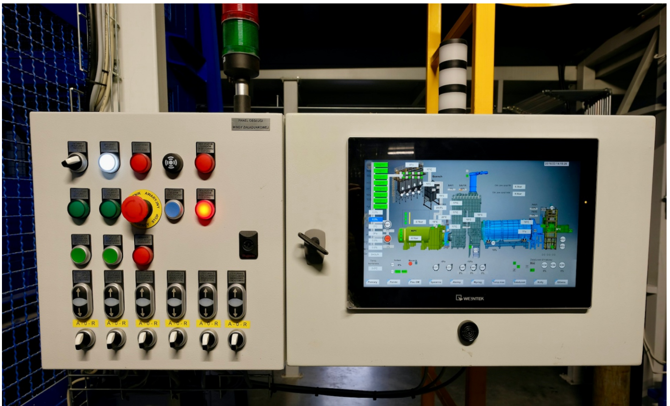
MONITORING AND VISUALIZATION AT EMKA S.A. IN KĘDZIERZYN-KOŹŁE - TECHNOLOGY HALL
