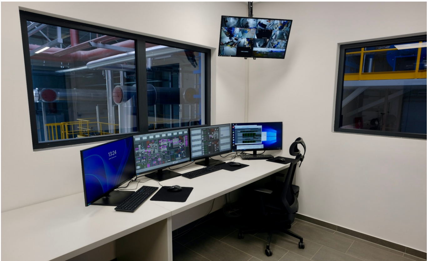
MONITORING AND VISUALIZATION AT EMKA S.A. IN KĘDZIERZYN-KOŹŁE - CONTROL CENTER
