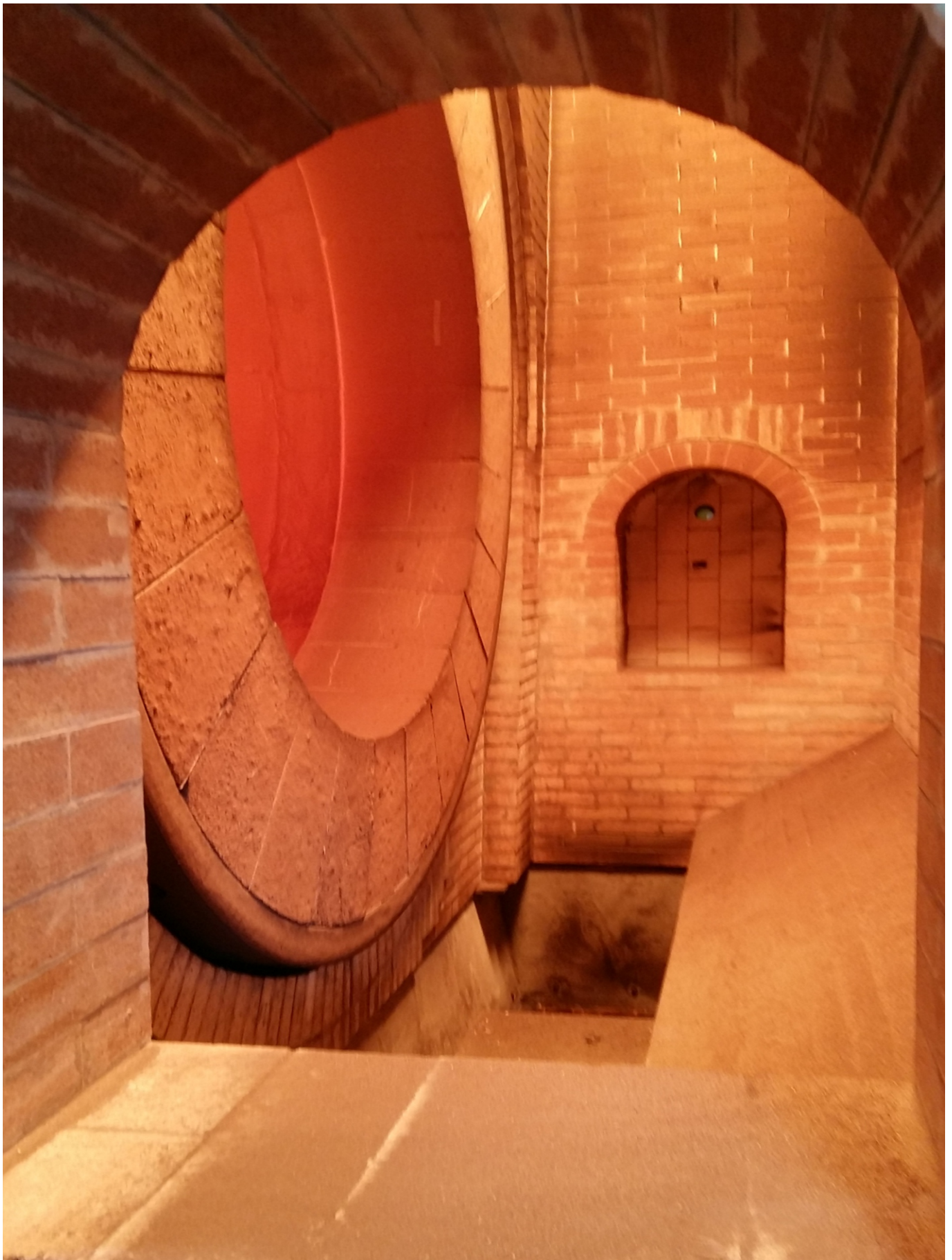
DISCHARGE CHAMBER INLET - CONNECTION OF THE ROTARY KILN WITH THE CHAMBER (INTERNAL VIEW)
