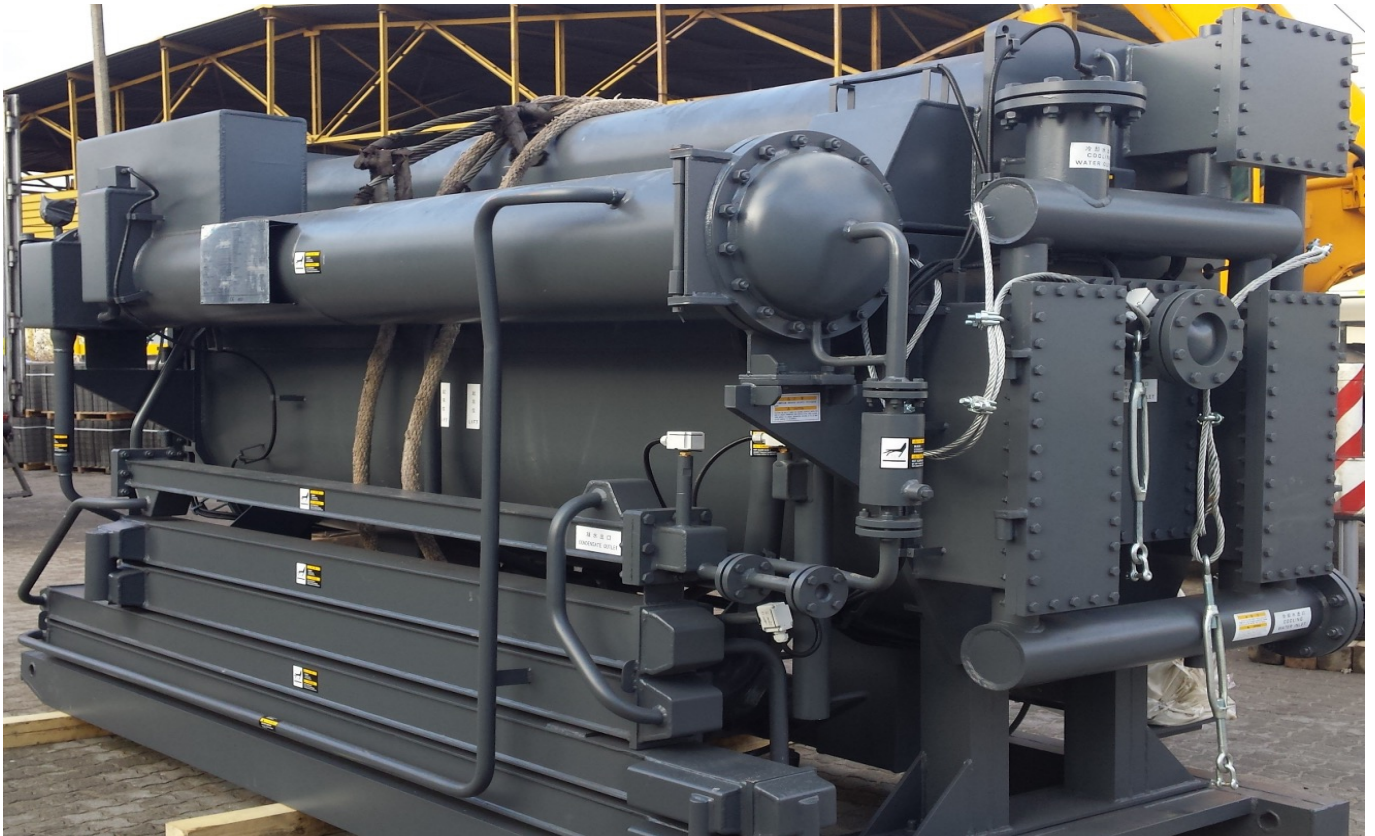
ABSORPTION CHILLER WITH Q = 0,6 MW
