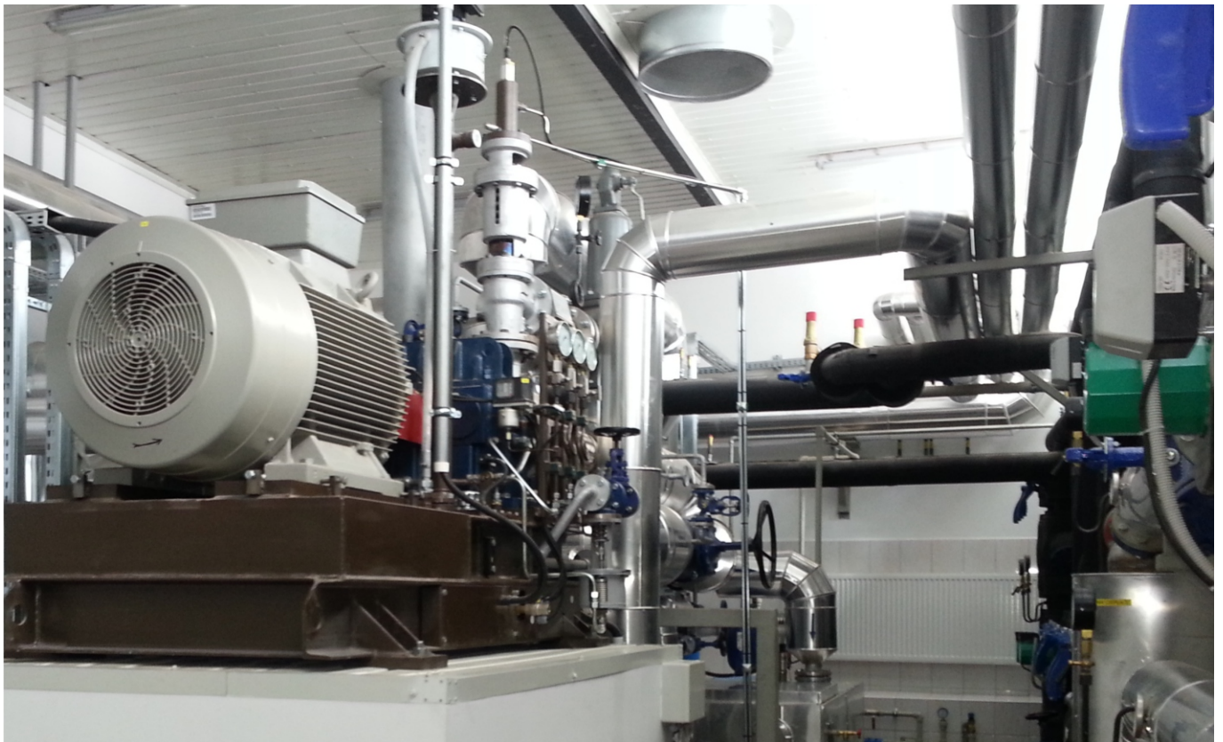
STEAM MICROTURBINE WITH N = 100 KWe
